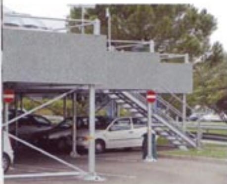
FastPark creates additional parking spaces in record time / FastPark schafft in Rekordzeit weitere Parkplätze
